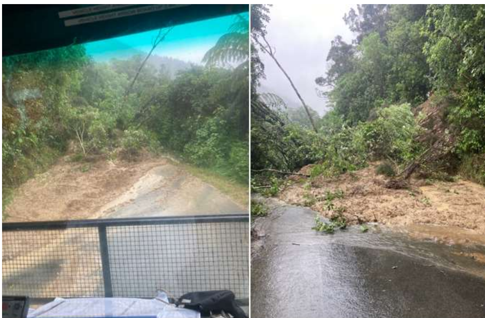
Figure 5: Kahuterawa Road December landslip
