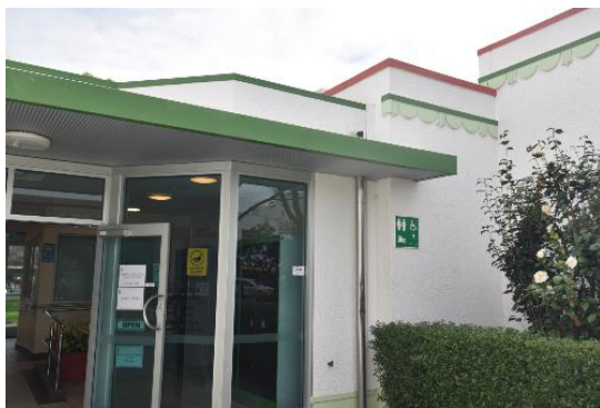
Figure 14 The junction between the rear of the Ladies’ Rest and the 2004 addition showing eastern entrance to the toilet corridor and I-Site complex. Anna Renton-Green, 25 September 2025, HNZPT.
